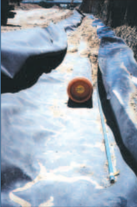
Jet fuel transfer line with blue PVC slotted conduit for TT5000 installed at a major international airport.
