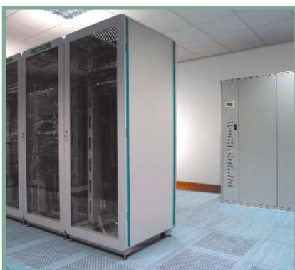
Data centre cooling
