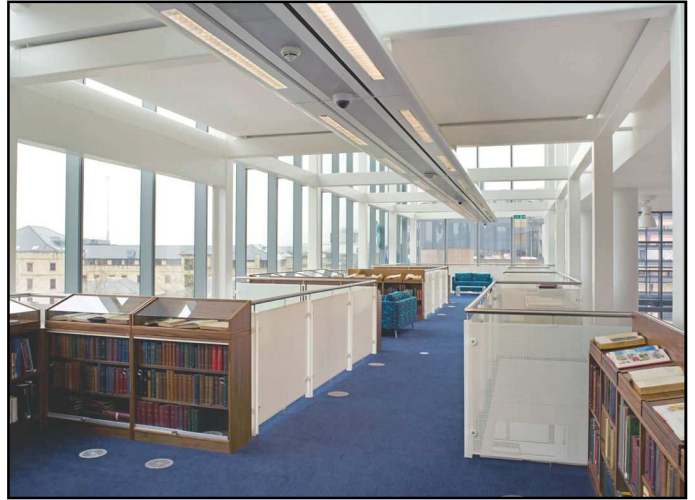
Multi Service Chilled Beam installed at Newcastle City Library
