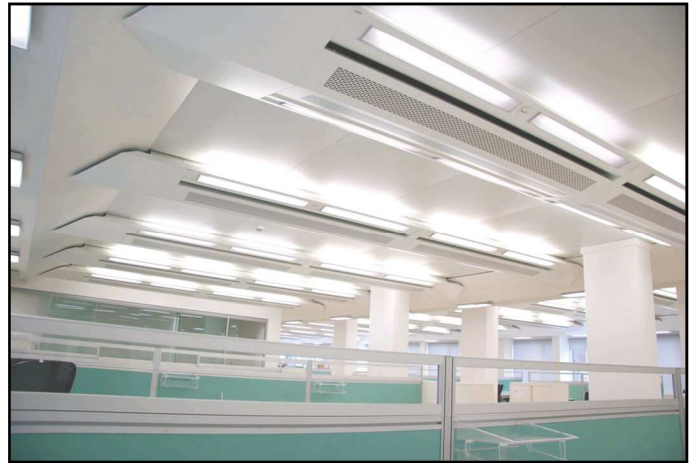
Active Multiservice Chilled Beam, 55 Baker Street, London
