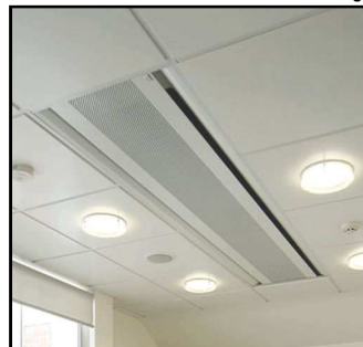
Active Chilled Beam in Ceiling
