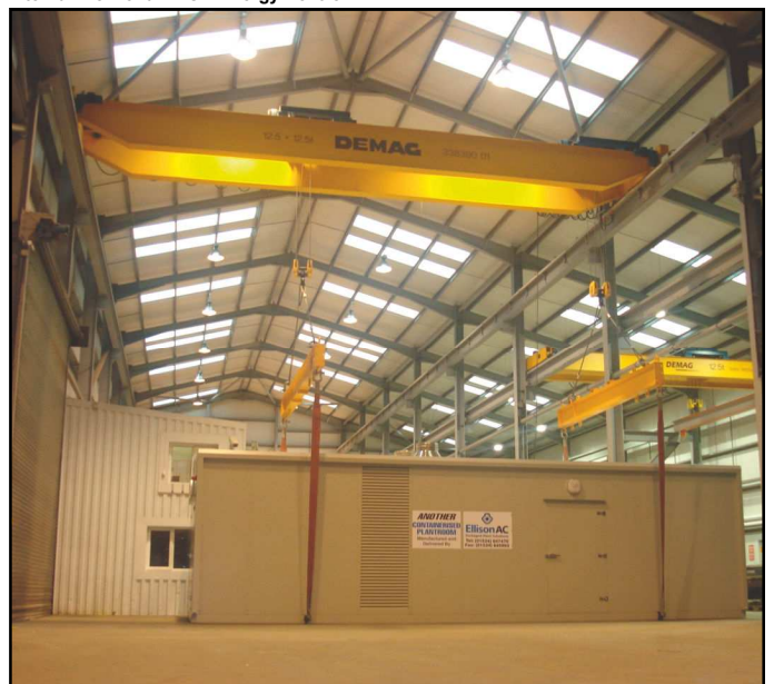
PlantPac Unit within Manufacturing Facility
