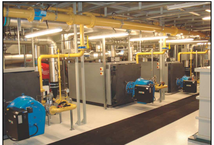
Internal View of an MOD Energy Centre
