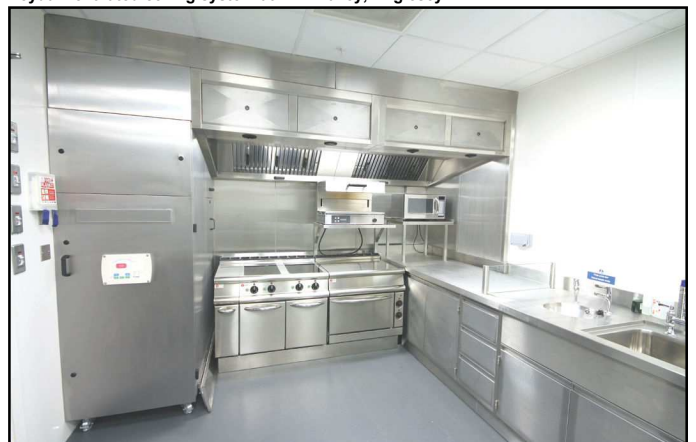
Refresh Self Contained System at Cadbury Green and Blacks, London
