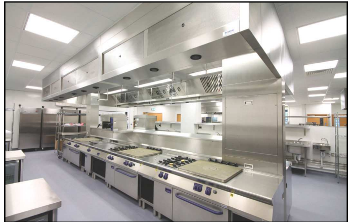
Ultrastream canopies installed at South Bristol Skills Academy
