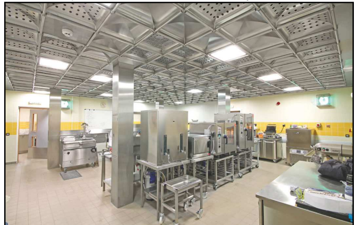
Heydal ventilated ceiling system at RAF Valley, Anglesey
