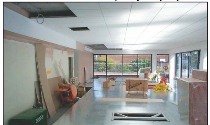
DURING refurbishment at The Center - Note the 100mm Ceiling Void & 300mm Floor Void
