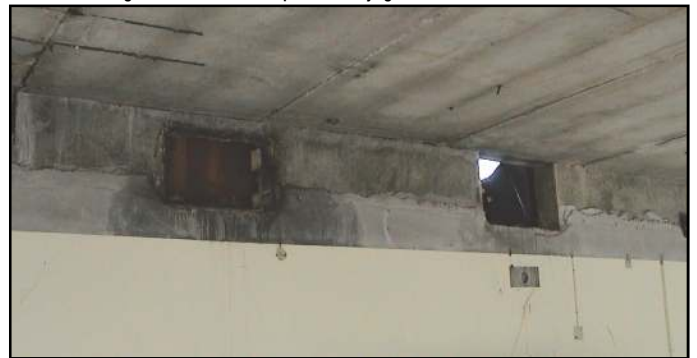
REFURBISHMENT at The Center - Gain this Headroom by Removing the Ceiling Ducting
